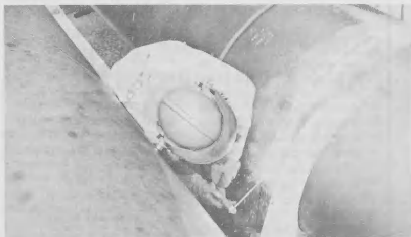
Sometimes the welders have to work in narrow areas as done here by Welder F. Soto.
